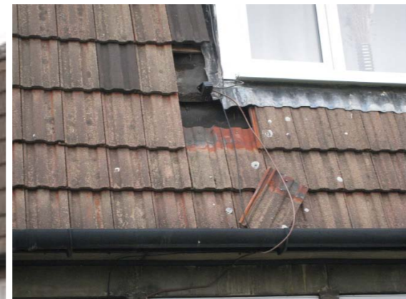
The old roof materials were causing a hazard.
